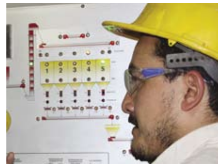
The 920i controls two bucket lifts, five conveyor belts, five in-motion conveyor scales and monitors levels in five silos.
