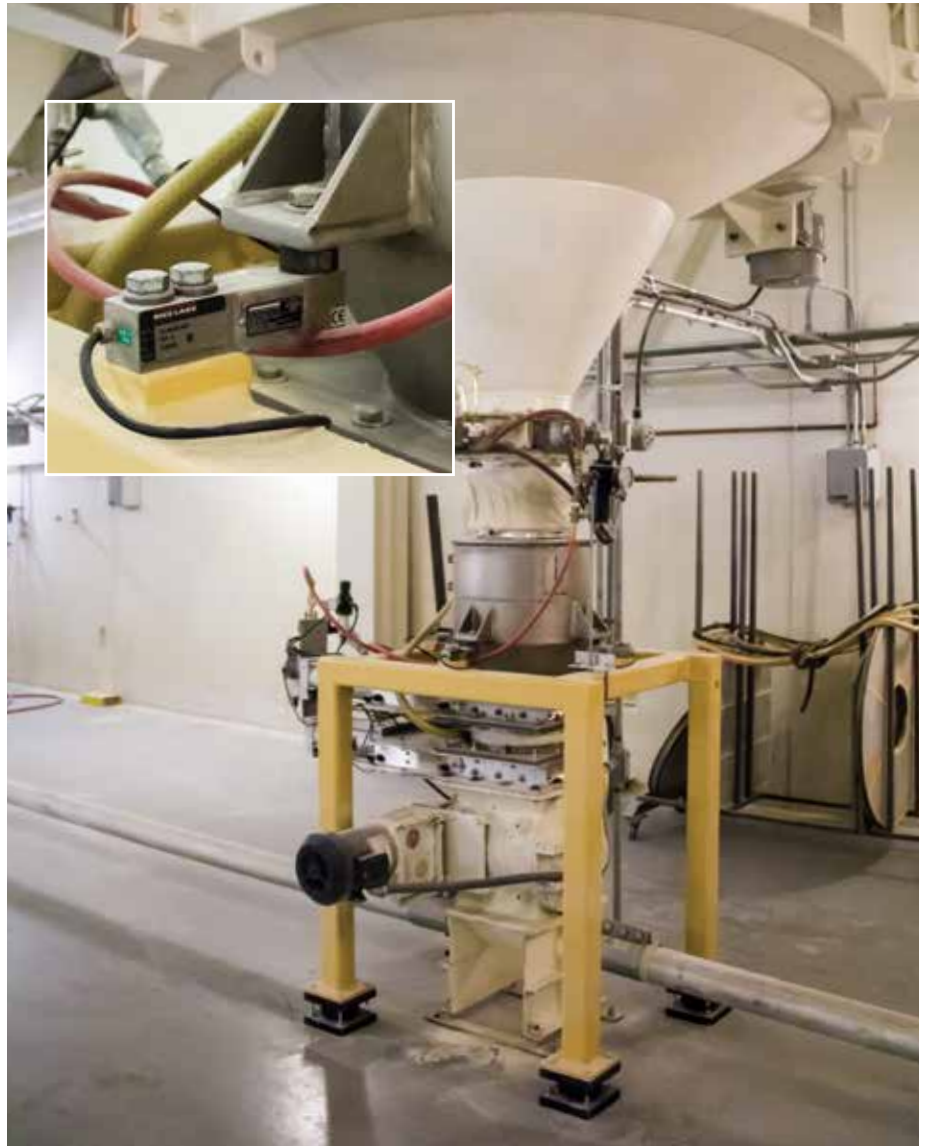
Semolina silos were outfitted with Rice Lake load cells to measure raw material usage.
