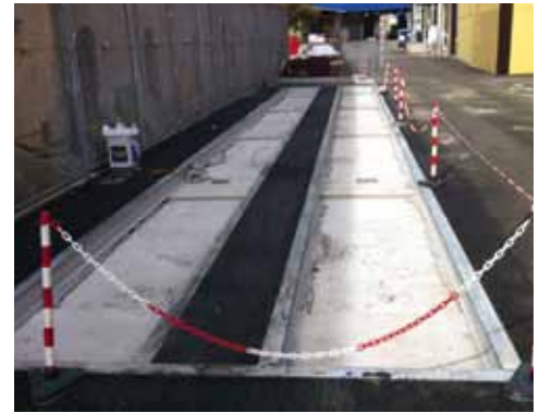
Example of an installation on an asphalt weighing surface
